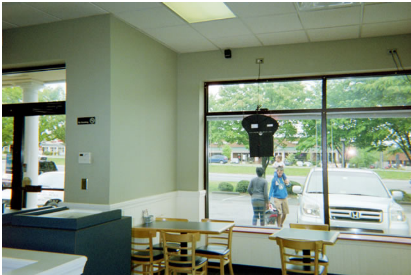
The mural and wood have been removed and as you can see large bubbles are present in the wall coating under where the mural had been
